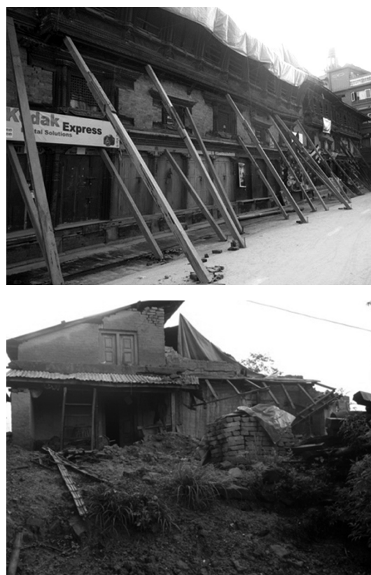
Figure 1: Buildings damaged by the earthquakes
